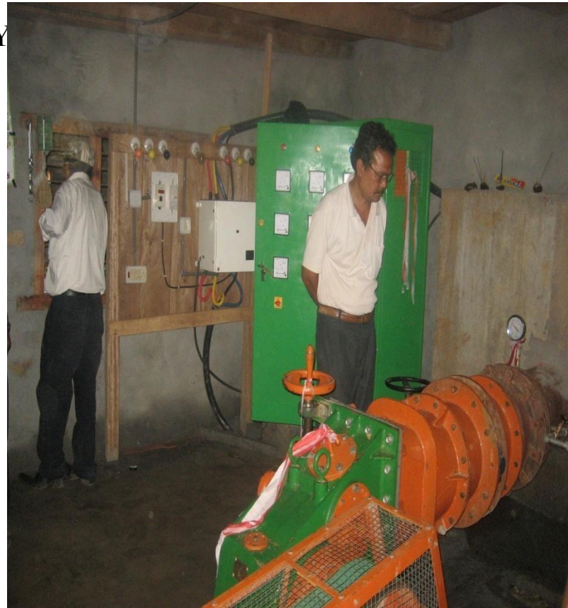
Inside view of MH powerhouse
