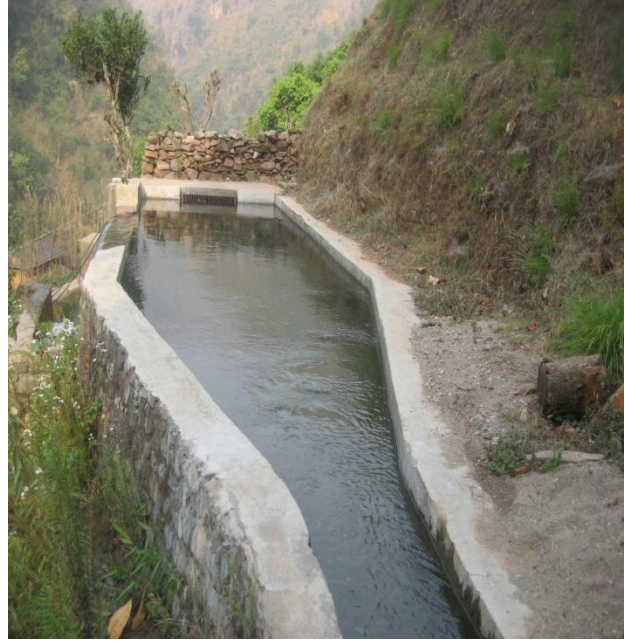
Forebay Tank of MHP
