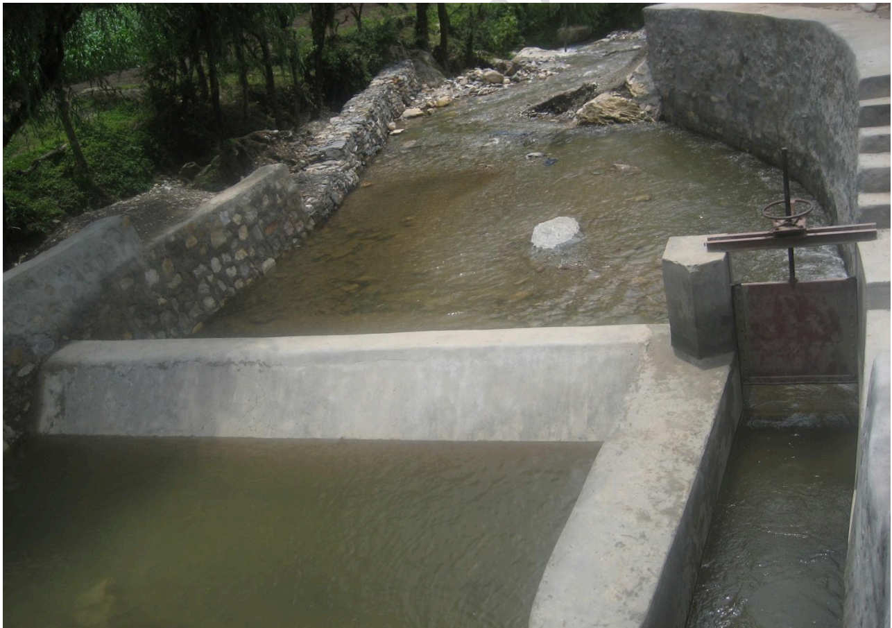
Intake Structure of Tara Khola Community Mini HEP (500 KW), Tara Baglung
